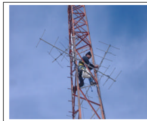
Figure 2. Assembling Yagi directional antennas on one of the towers of the array.
